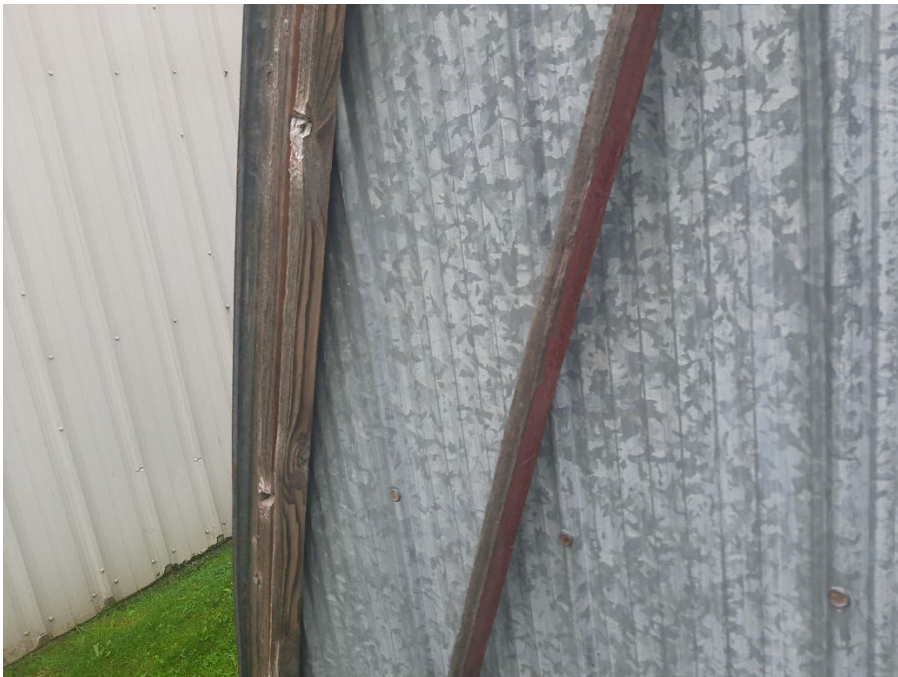
Photo 2 – Lead-based red paint on exterior wood trim.
